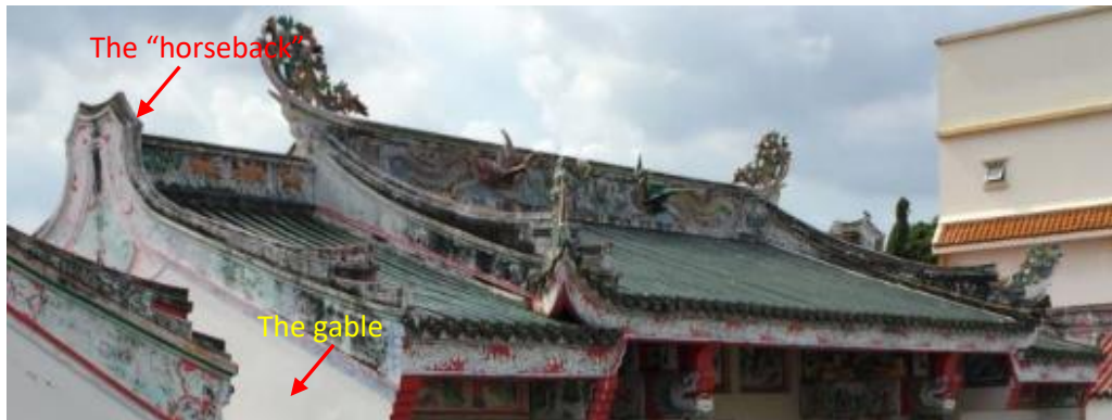
Figure 20 The three Chuan flush gable roof(硬山三川屋顶) of the head door's roof
