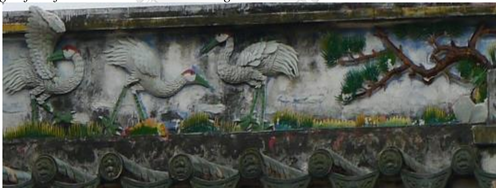
Figure 22 The Chaozhou trencadís of the cranes and pine trees in the left ridge abdomen
