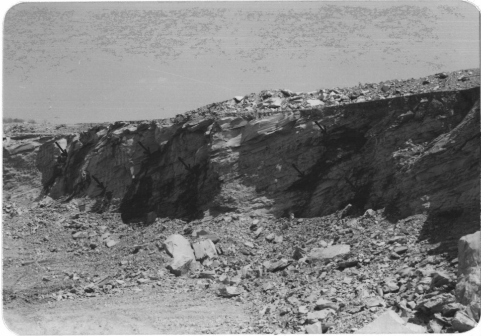
Figure 10. Water seepage along bedding in Subarea 5 (at the arrow).
