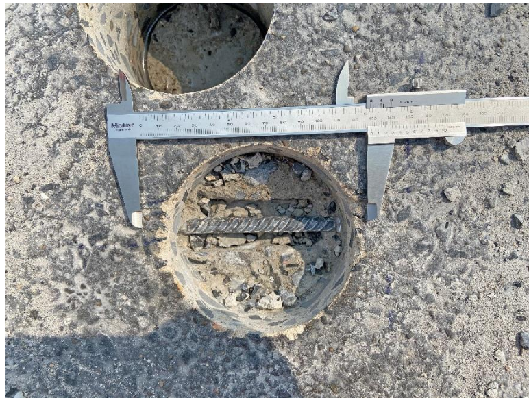
Figure 85 Steel surface on bridge span no. 5 at gridline N-O/5
