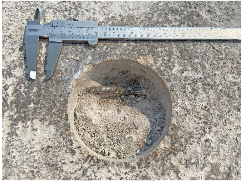
Figure 87 Steel surface on bridge span no. 9 at gridline E/4
