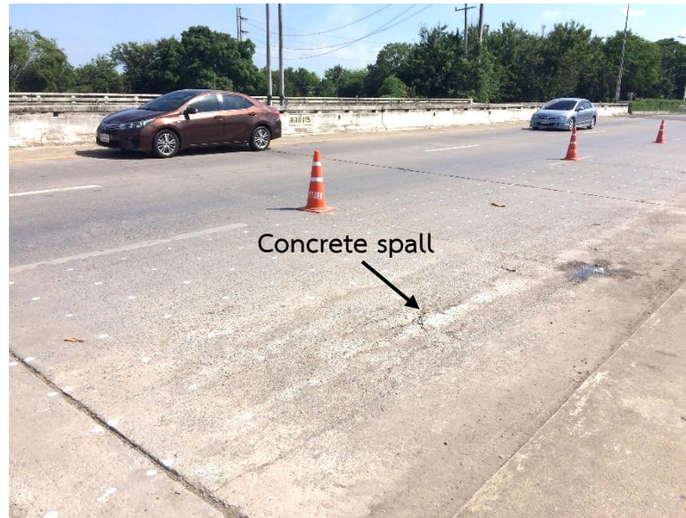
Figure 16 Concrete scaling on along wheel path
