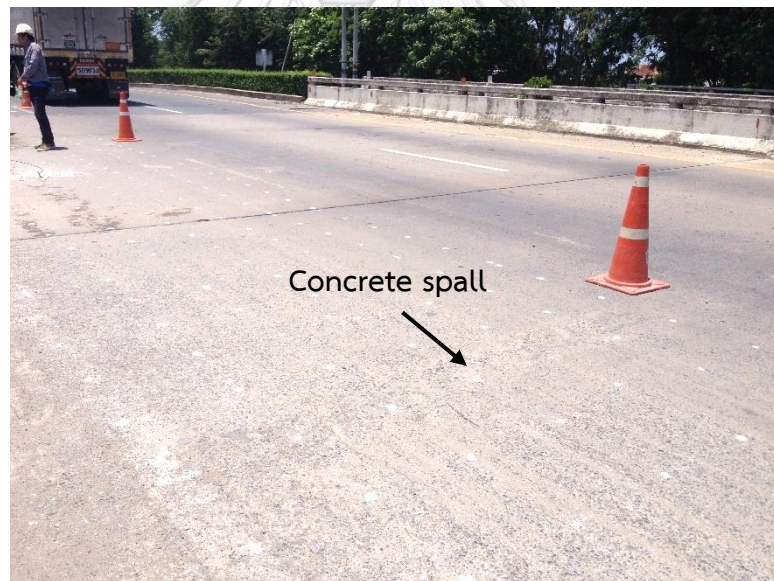
Figure 15 Concrete spall on the middle bridge span
