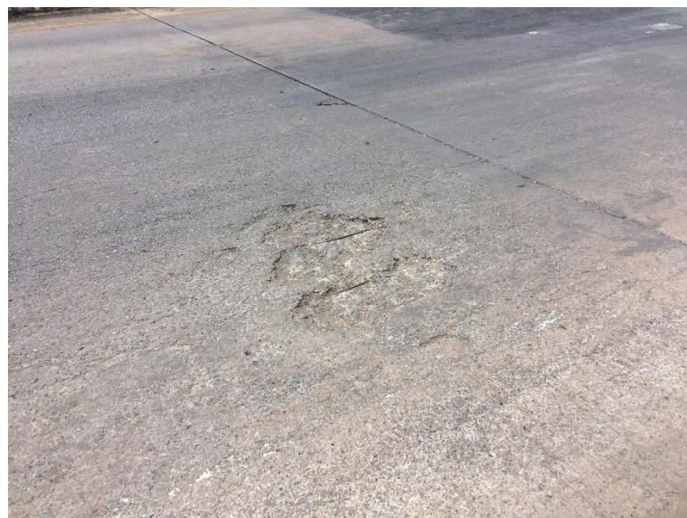
Figure 13 Concrete spall until reinforcing steel level
