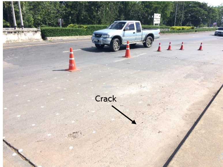
Figure 14 Longitudinal and transverse cracks on bridge deck
