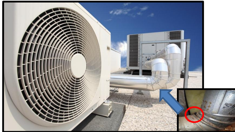
Figure 19 Duct leak in air distribution system
