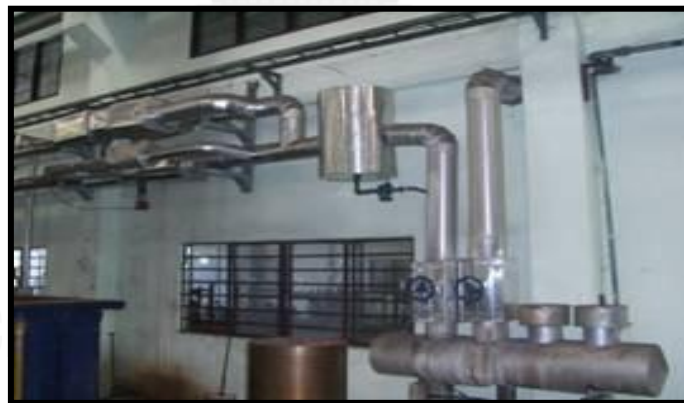
Figure 42 Insulation of steam distribution pipe
