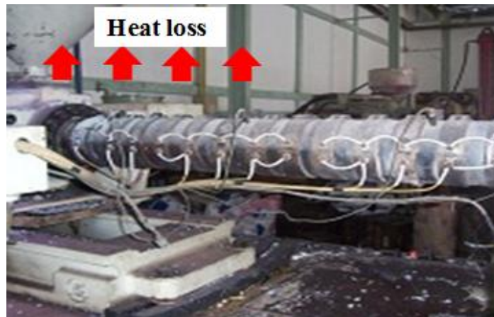
Figure 25 Heat losses in an extruder machine
