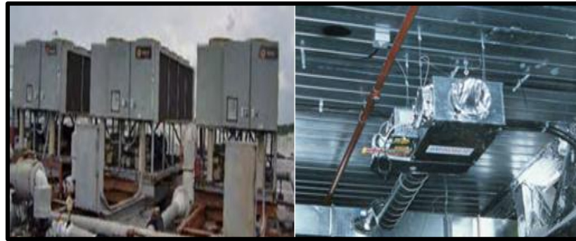
(a) Outside air conditioning system (b) Inside air conditioning system
