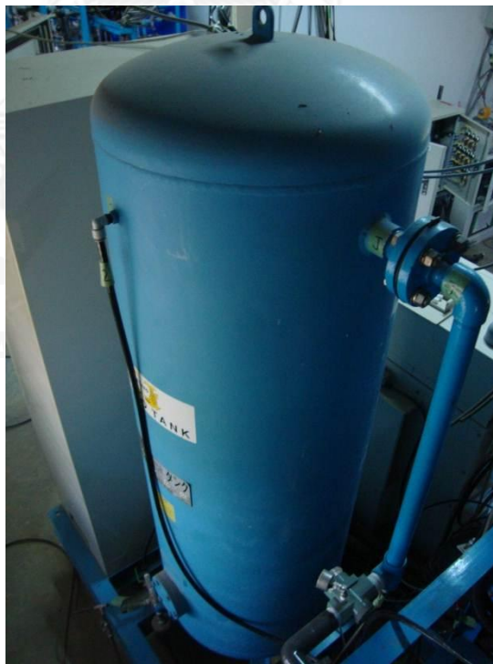
Figure B. 5 Pressure Tank
