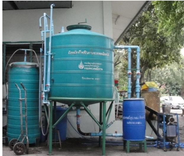
Figure 2.4: Anaerobic digester pilot plant in Sathya Sai School Thailand
