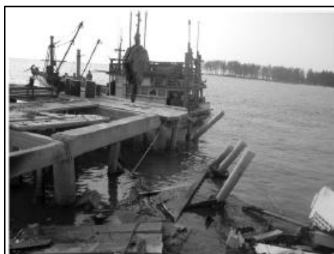
Figure 1.1 Damage to Khao Lak Harbor (Saatcioglu M. et al. 2006)
