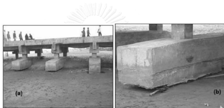
Figure 2.11 (a) Substructure of the jetty at Colachal harbor, in Kanyakumari; the jetty remained intact. (b) Close-up of the jetty foundation, which was resting on piles. (Makeshwari B. K. et al., 2006)
