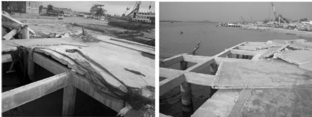
Figure 1.5 Damage to precast slab strips of the concrete dock in Khao Lak Harbor
