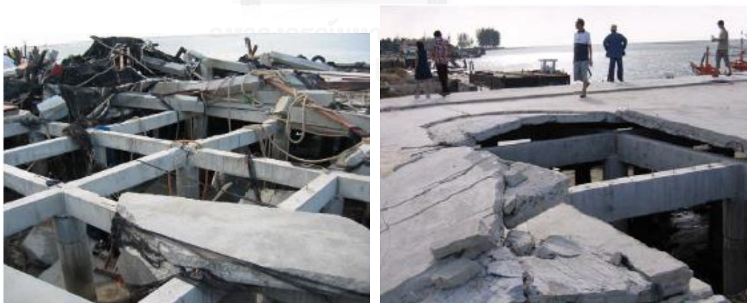
Figure 1.4 Damage to pier deck on Ban Num Kem Port, (a) joint failure, (b) failure of precast concrete slabs (Lukkunaprasit Panitan, and Ruangrassamee Anat ,2008)
