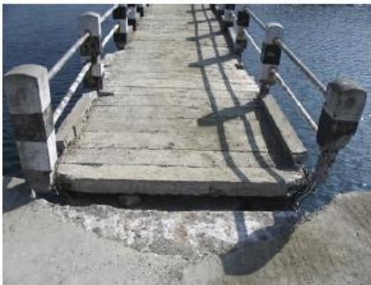
Figure 2.37 Pounding damage to jetty at Sagar Dweep. (Goutam Mondal, Durgesh C. Rai, 2006)
