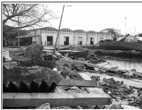
Figure 2.10 Damage to the quay in the innermost area of the Galle Port. (Tomita T., et al. 2006)
