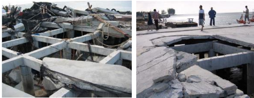
Figure 2.12 Damage to pier deck on Ban Num Kem Port, (a) joint failure, (b) failure of precast concrete slabs (Lukkunaprasit Panitan, and Ruangrassamee Anat ,2008)
