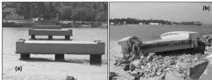
Figure 1.3 Damaged Keelamanakudy Bridge on the Palyar River: (a) substructure of the bridge all four spans washed away; (b) a span that washed about 20 m away. (Makeshwari B. K. et al., 2006)
