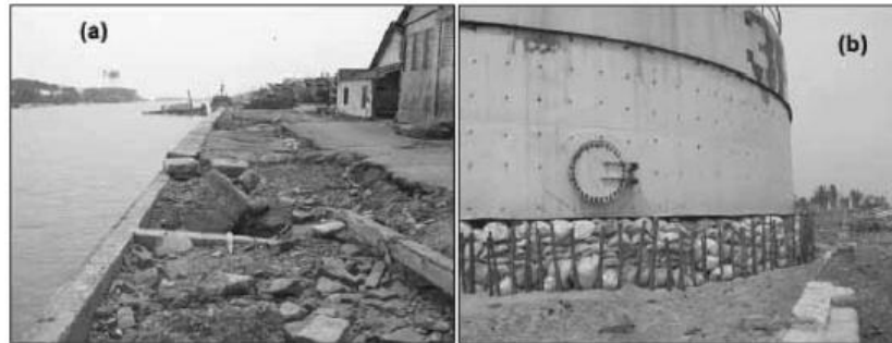
Figure 1.2 (a) Damage to a wharf at the Nagapattinam harbor. (b) Base of an oil tank damaged by erosion; sandbags were temporarily placed to support the tank. (Makeshwari B. K. et al., 2006)
