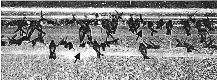
Figure 5.2. The supporting wood (dark arrows) attached on the smooth wall under the ceiling in the sacred building of Suthiwatwararam Temple, Samut Sakhon Province.
