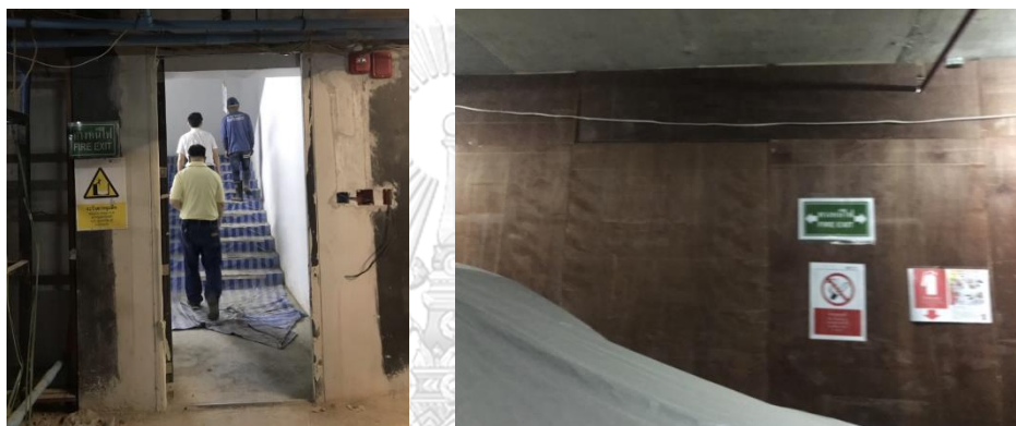
Figure 4.6 Fire exit signs in construction project number 2 and project number 6
