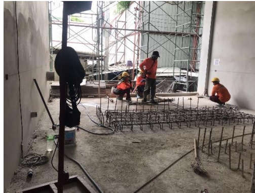
Figure 7.31 Example of the number of construction workers on day 2 in the construction project.
