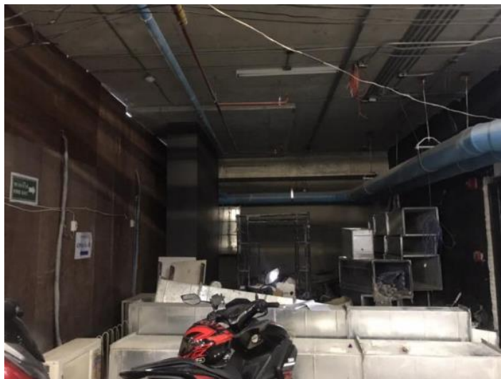
Figure 1.2 An object obstructed by materials and equipment in the construction project.
