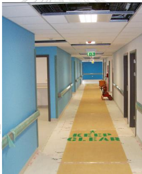
Figure 2.1 Keep fire exits clearly signed and free from obstructions (HSE, 2010)
