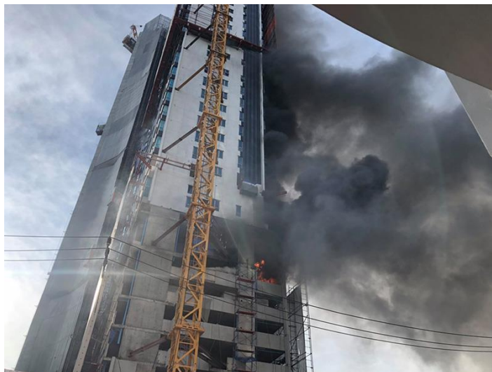
Figure 1.3 Fire accident at the construction project (JS100 Radio, 2021)
